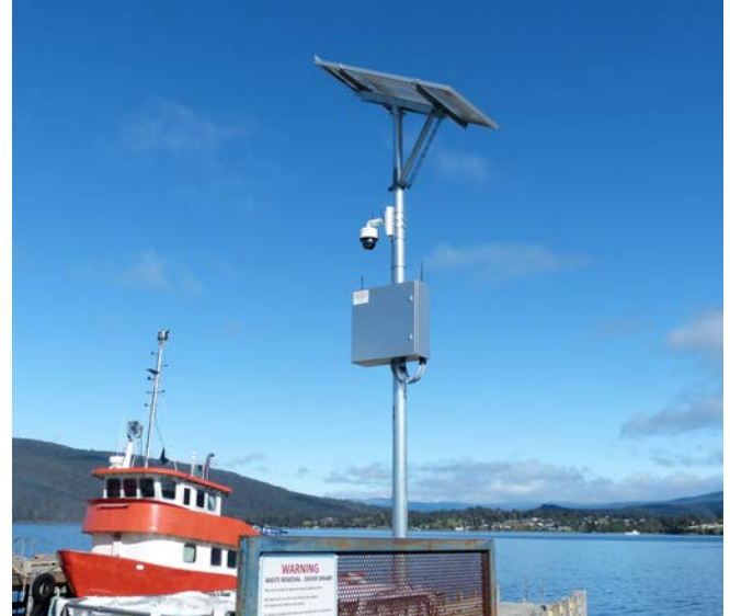
CCTV Camera Dover Jetty
