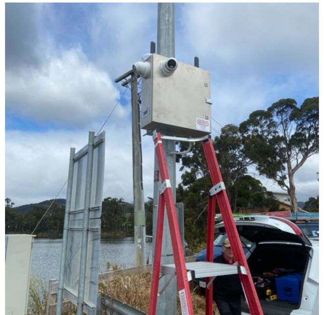
CCTV Cameras on MAST Facilities
