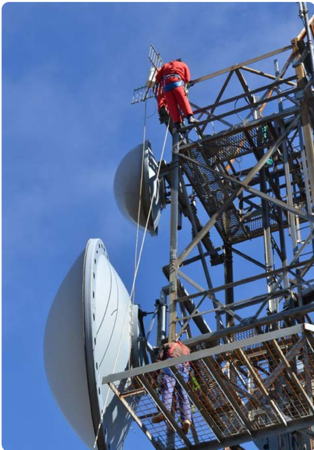
Riggers at the top of the Mt Read tower installing a robust radio link antenna for this extreme environment. This is to control the Elliot Range base.
