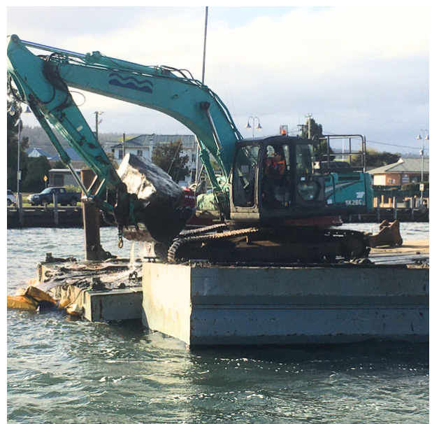
Large sandstone boulder being removed from between the boat ramp and main wharf
