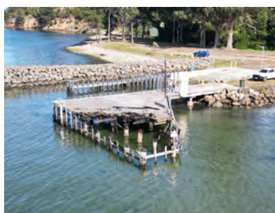
Damage at Gordon Jetty
